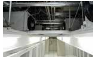
Ceiling-suspended air conditioning
