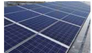
Photovoltaic power generator
